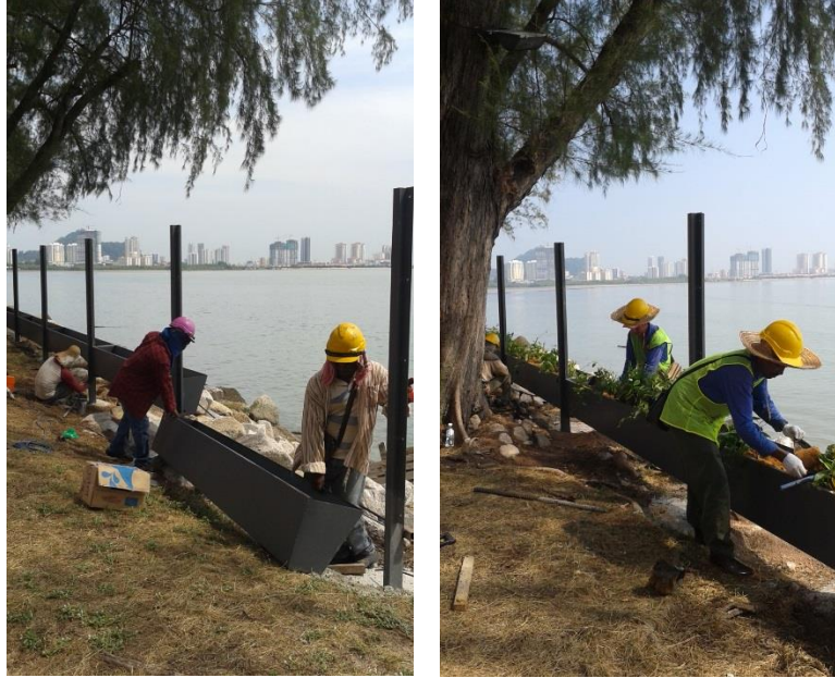
(Left) Mounting of planter boxes continue at the latest section of fencing installation works; (Right) Workers ensuring the creeper plants are planted properly
